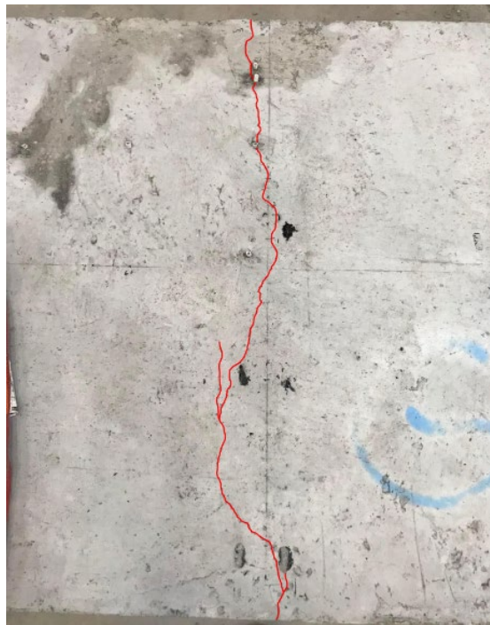
Figure 5.17 Cracking in concrete of Panel 1, at top concrete surface
