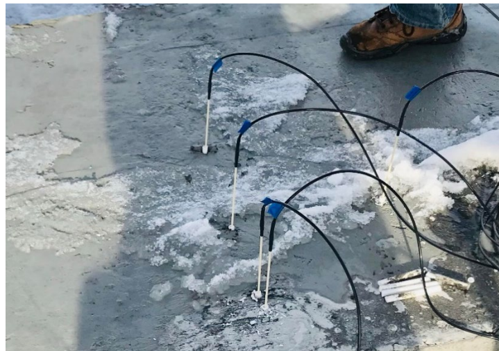
Figure 3.14 Temperature sensors inserted into the tubes
