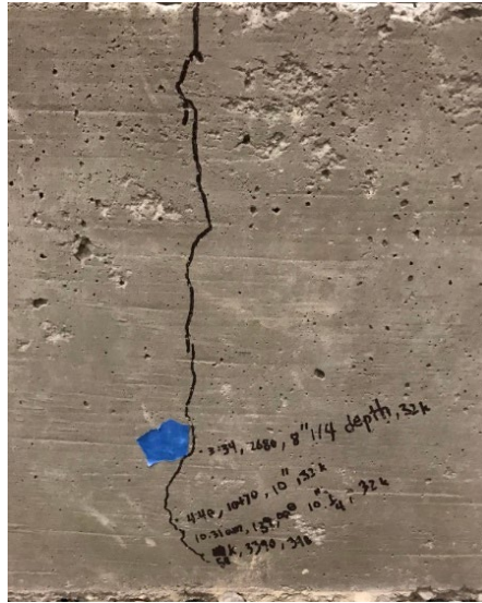
Figure 5.20 Cracking in concrete of Panel 2 at side
