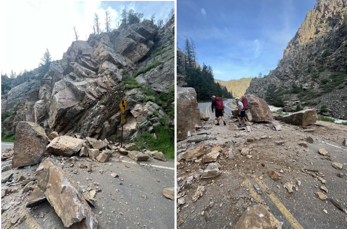
Figure 3.1 Rockfall damage on Highway 14 on June 9, 2023, at 6 AM. The PI and colleagues (right) were on scene to investigate the level of damage and attempt to image the resulting starting and final position of the rockfall. The highway was closed for about four hours, but after an incredible response by CDOT was shortly reopened despite significant damage to the surrounding asphalt.
