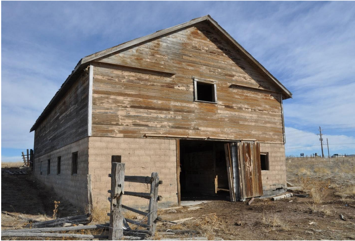
Figure 2.11 A historic barn structure used to examine the accuracy of the SfM methodology for a relatively simple geometry.
