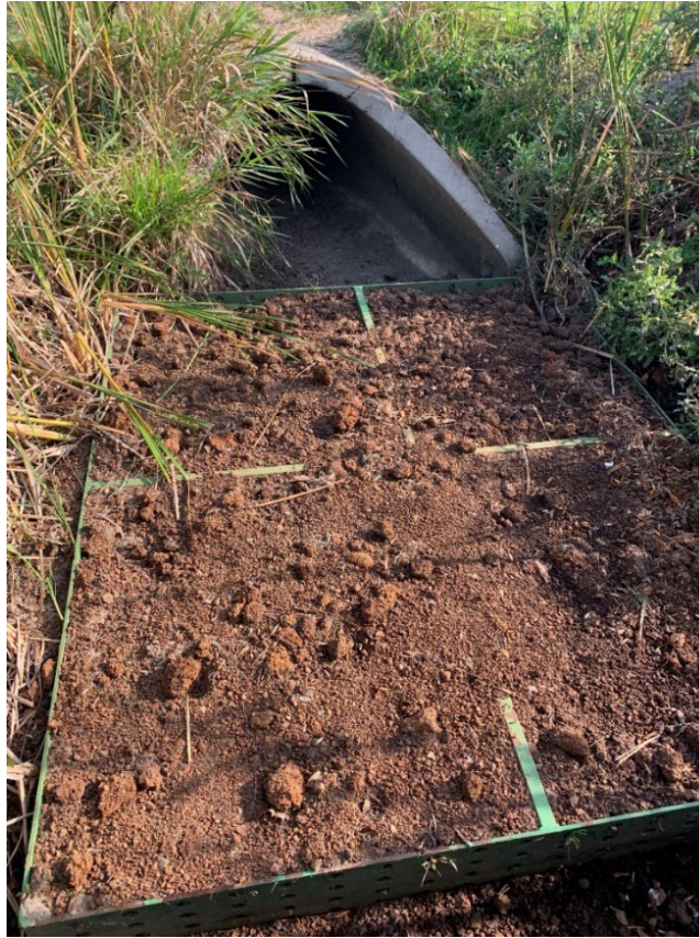
Figure 2.7 Filter material agglomeration observed during the field study
