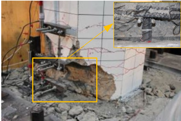
(c) At the end of test (cracks, spalling, fractured rebar, and exposed rebar cage.)
