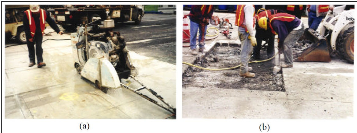
Figure 2.2 (a) sawing the repairing boundaries and (b) removing the repairing area using jackhammer (Wu et al. 2001)
