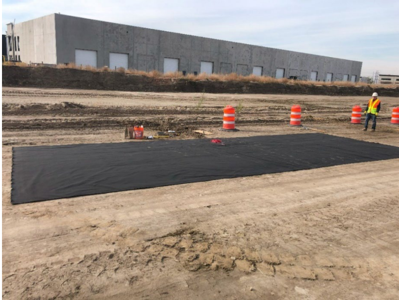
Figure 3.15 One of the 37-foot instrumented sections of geotextile installed on the subgrade
