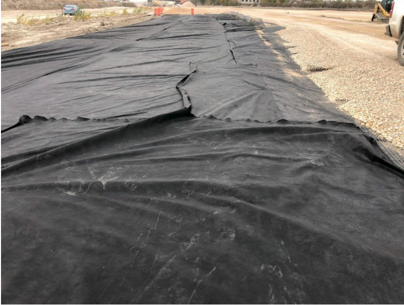
Figure 3.17 Photo of geotextile installed on the subgrade with folds and uneven overlap
