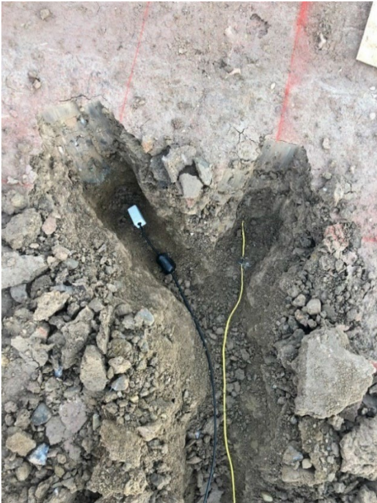
Figure 3.14 Photo of moisture and temperature sensor installed in the subgrade
