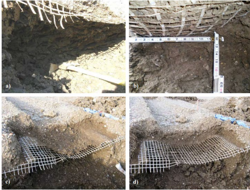
Figure 2.4 Inspection of geogrid after experimentation in the field (Cuelho & Perkins, 2009), courtesy of Western Transportation Institute and Montana State University - Bozeman
