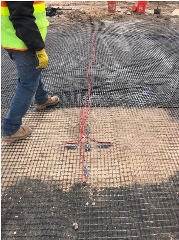
Figure 3.16 Photo of geogrid with strain gages installed on top of the geotextile in S4 as part of the geocomposite
