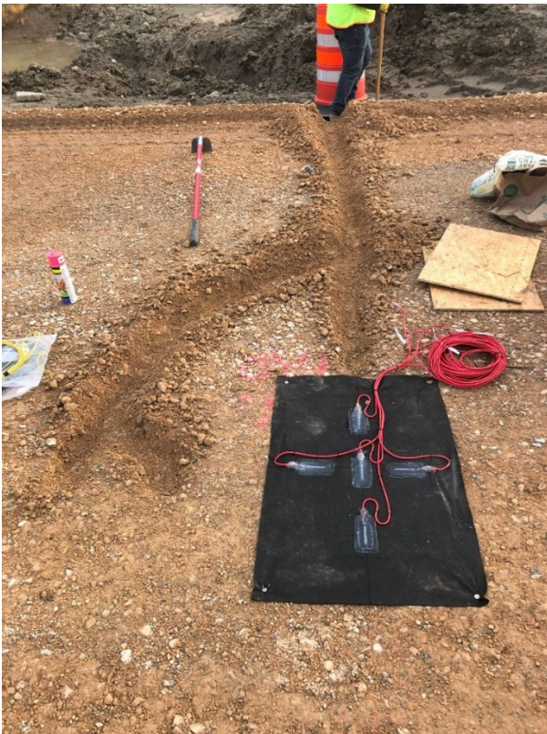
Figure 3.20 Trenches dug for the installation of the moisture and temperature sensor two feet and three feet down station from the strain gage array at location 2A
