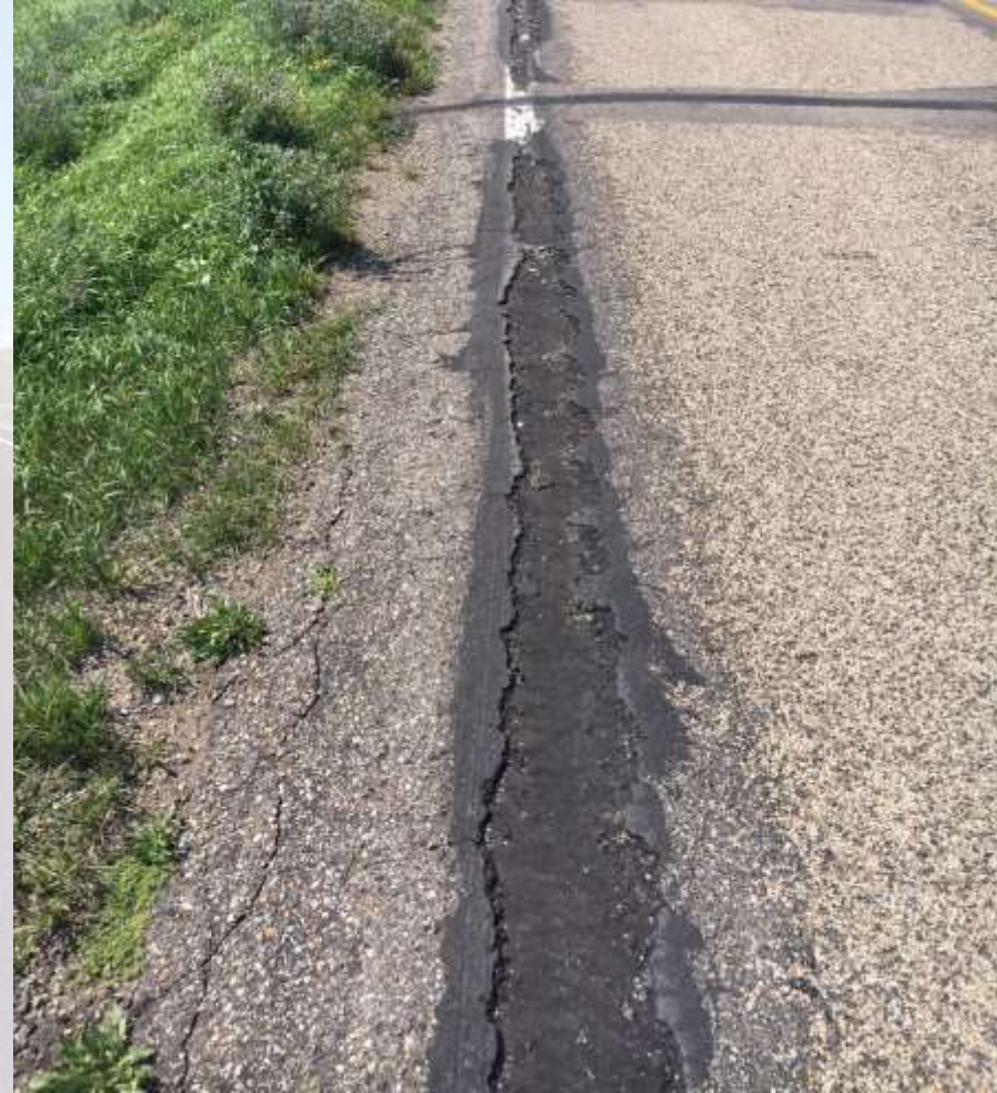
Rumble Strip Degradation
