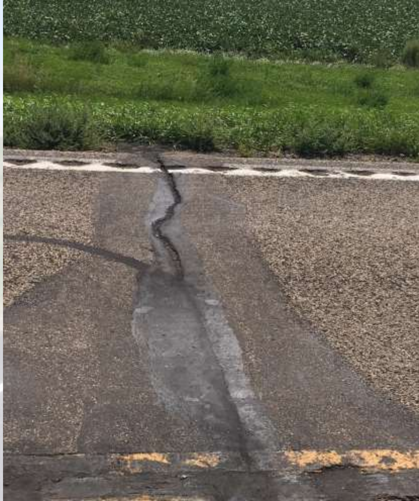
Thermal Reflective Cracking
