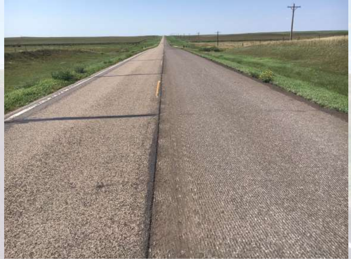
After Sweeping – transverse cracks barely noticeable
