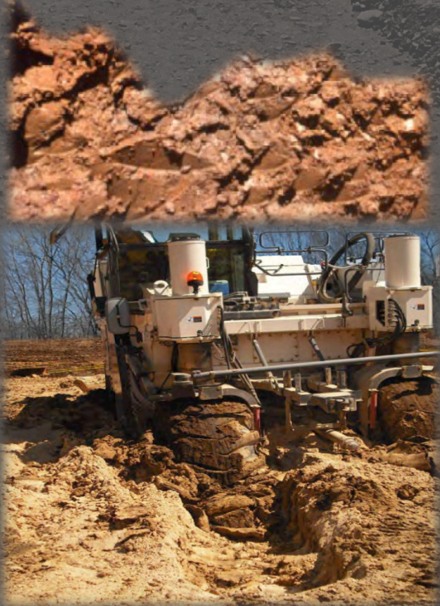
Unstable Wet Subgrade
