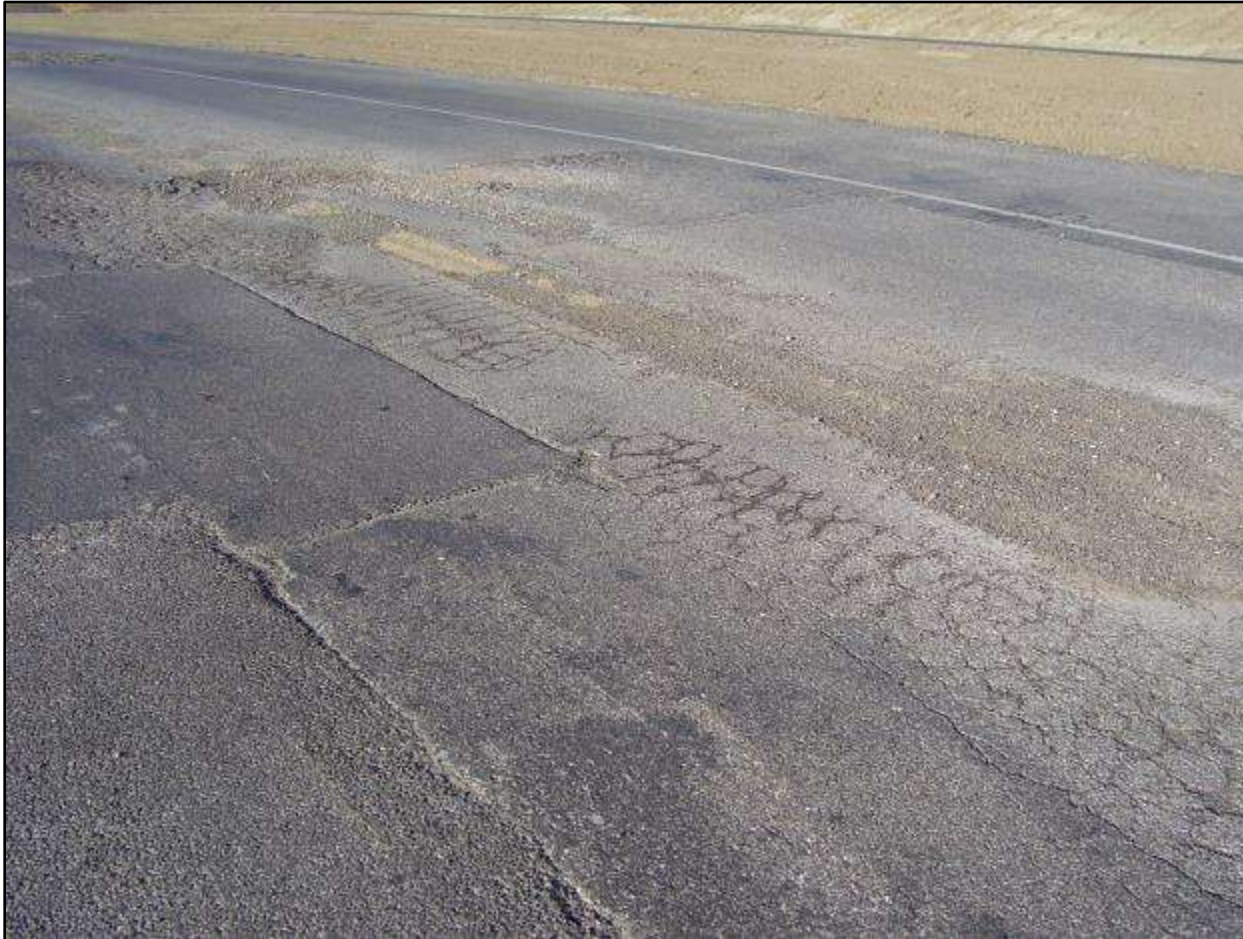
Alligator cracking on ND Highway 23 near Johnson's Corner between Watford City and ND Highway 73.
