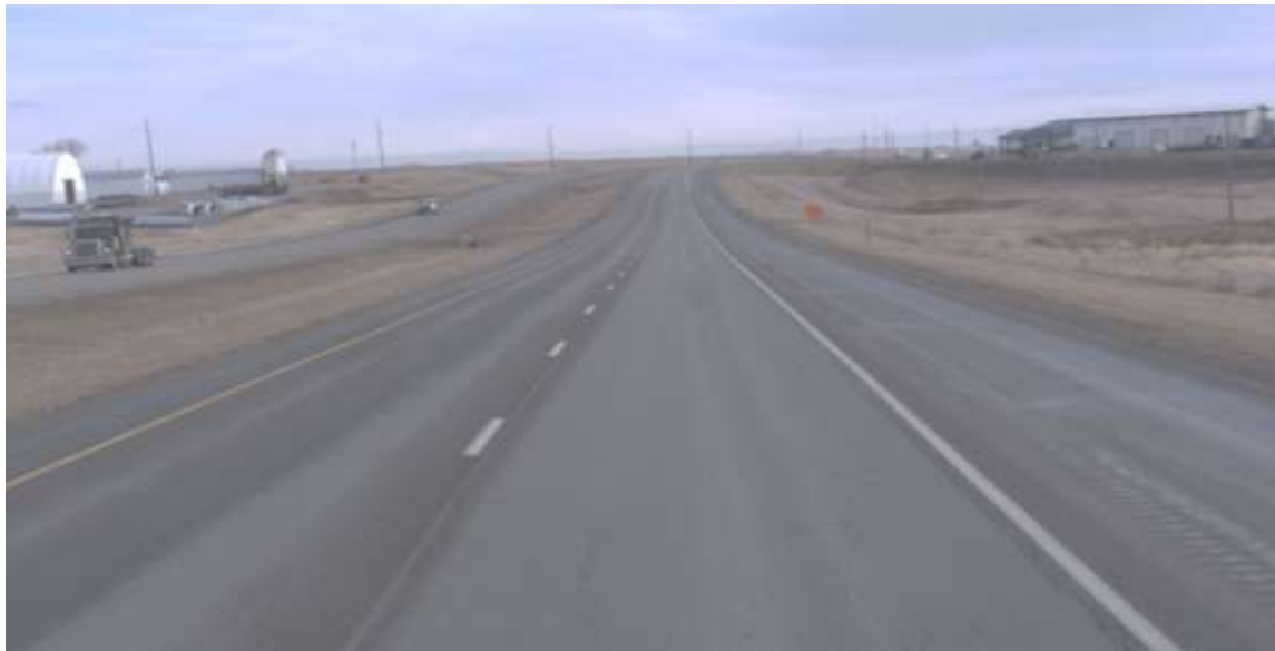
Rutting on US Highway 2 Eastbound Stanley to Palermo.
