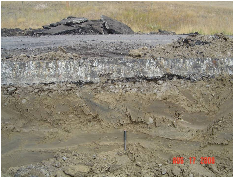
5" Asphalt, + 6" Base (15 yrs old)
