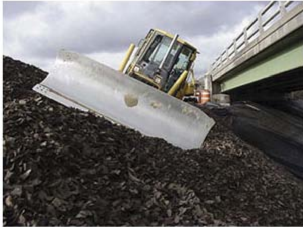
A bulldozer is leveling a pile of shredded tires that are being reused as lightweight fill for a bridge abutment and slope. Recycling is one aspect of creating greener highways.
