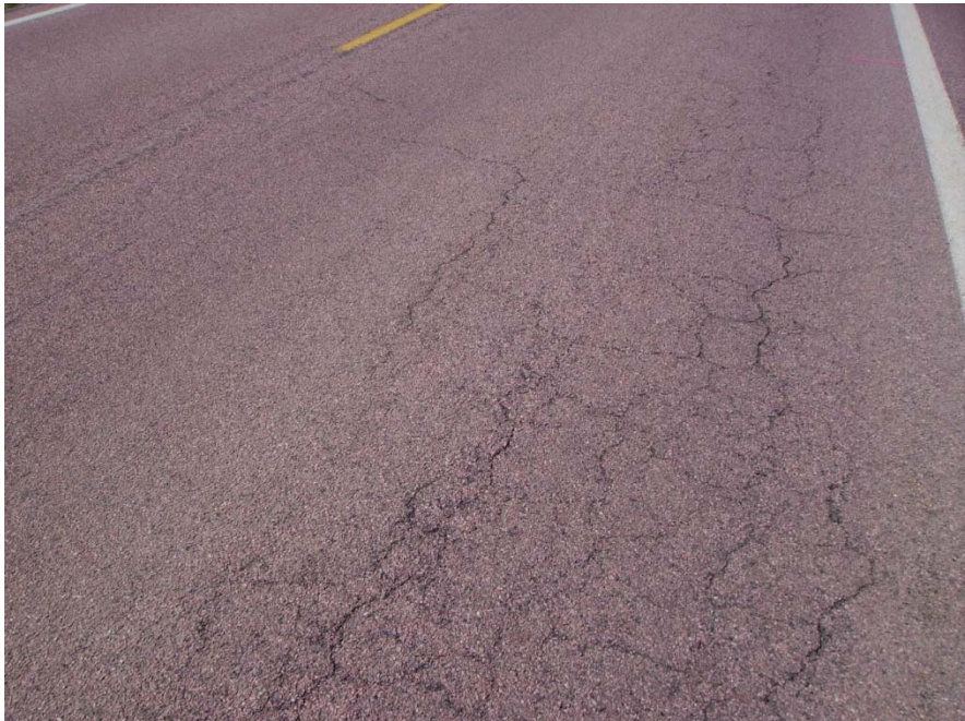
Fatigue Cracking Section SS2
