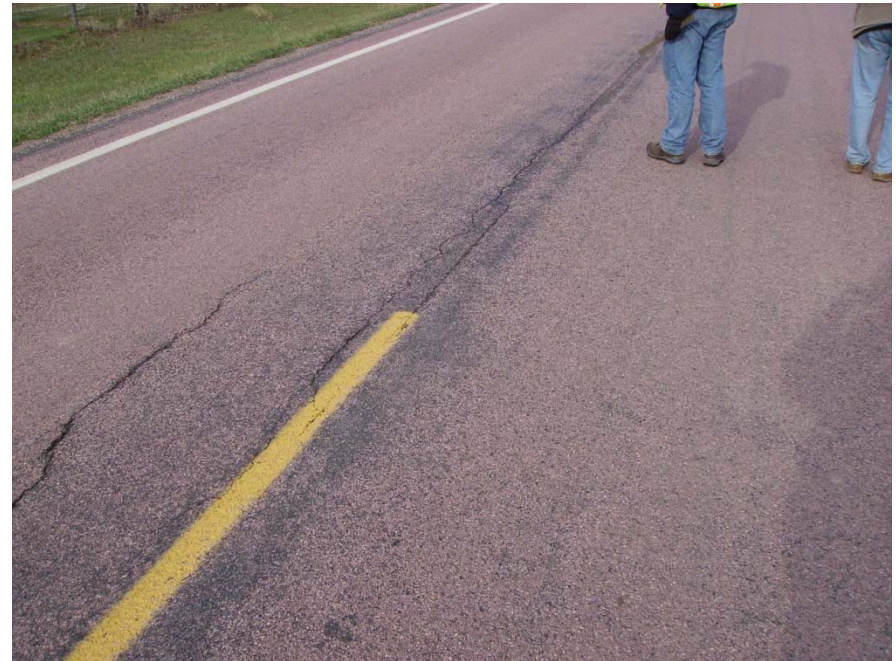
Longitudinal and centerline cracking
